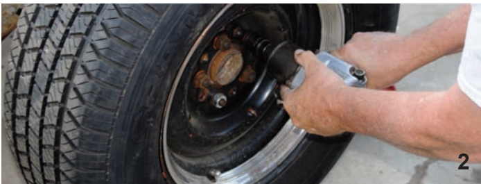
The lug nuts were disconnected with an impact gun that was outfitted with the correct size socket. Before the tires were removed, the chassis was elevated with a floor jack and then the frame was supported by large jack stands.
