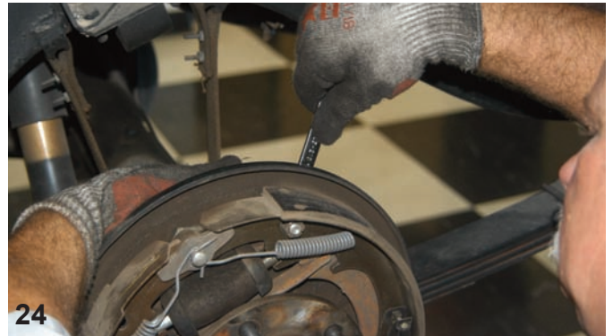
Using a long box-end wrench the bolts that connect the backing plate to the axle were removed.
